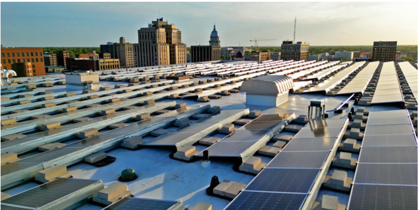
Solar panels on the roof of Horace Mann’s headquarters building in Springfield, Ill.
